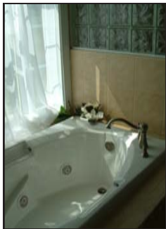
Virginia Class A Contractor - Master Plumber and Gasfitter - Certified in Radiant Heat, Wardflex and Backflow Prevention
